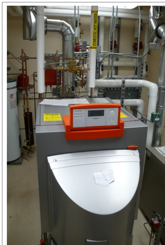
This boiler has separate pipes for hydronic distribution and domestic hot water.
