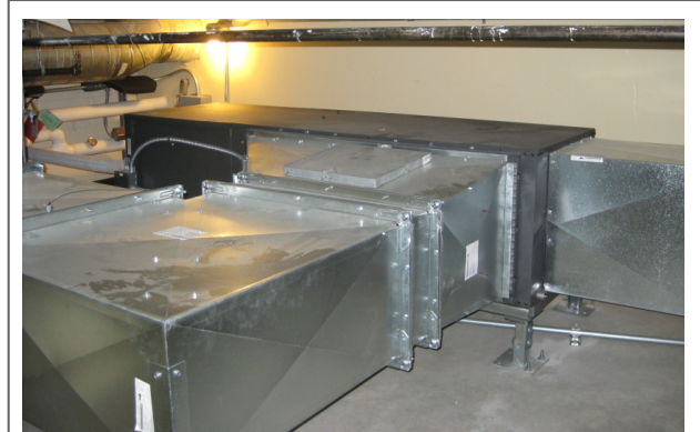
Air ducts take heated air to and from a ground source heat pump.
