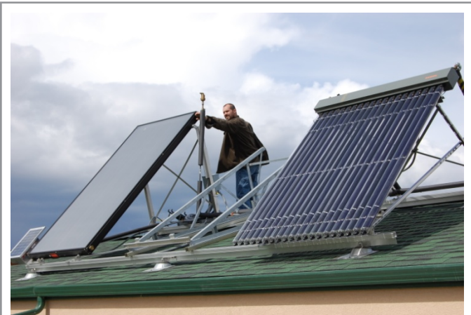
Flat-plate collector (left) and evacuated tube collector (right) on a south-facing roof.
