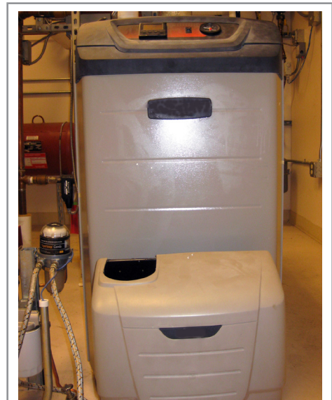
A boiler produces heated water or steam.
