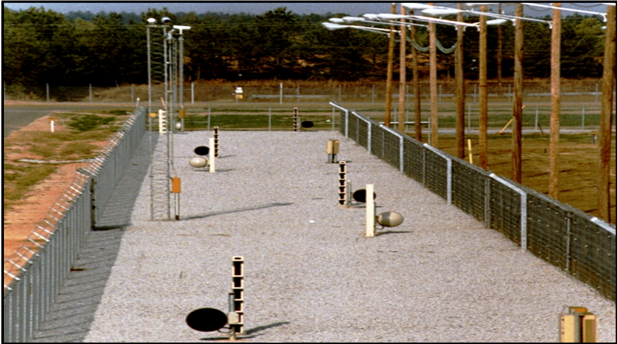
Figure 2-7b: Double Fence Line
