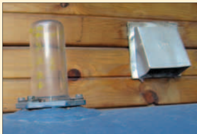
Oil level gauge. Note the empty tank.
