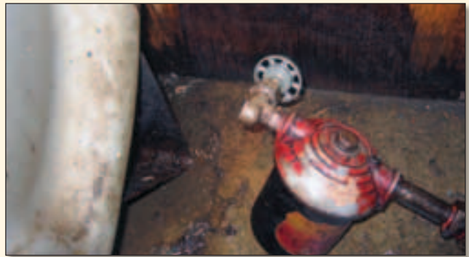
Broken valve on oil tank in basement.
