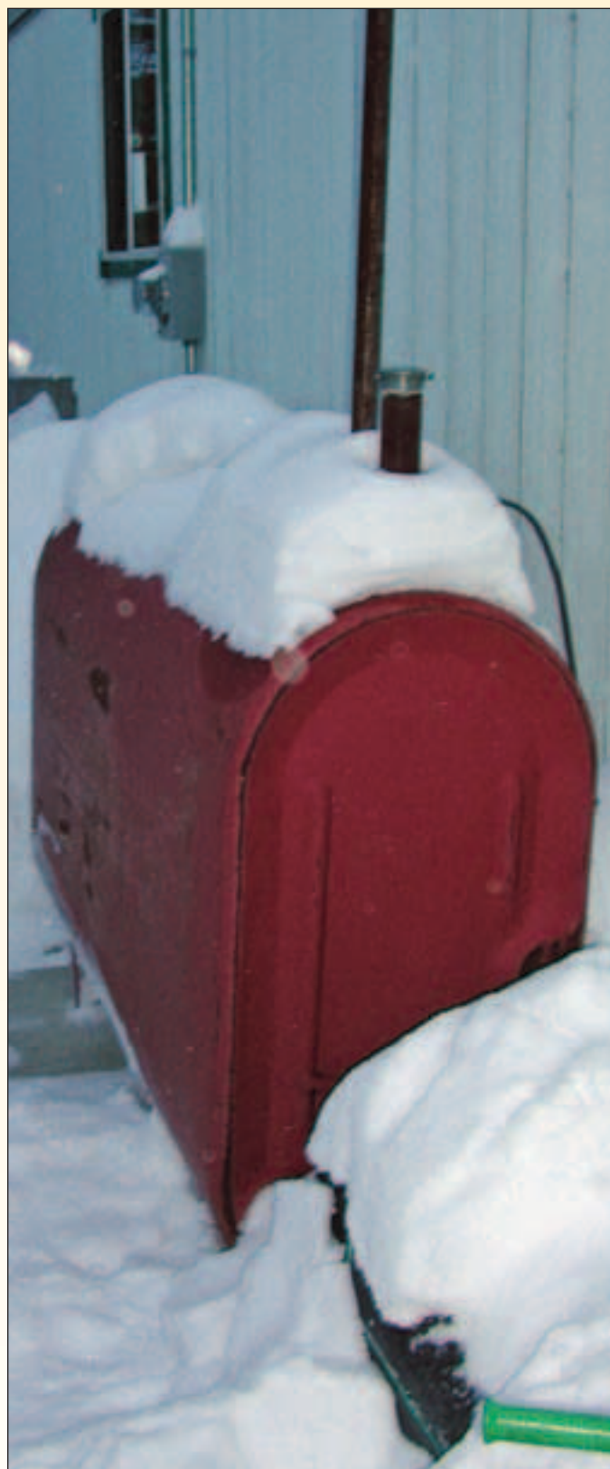
Typical oil tank location.
