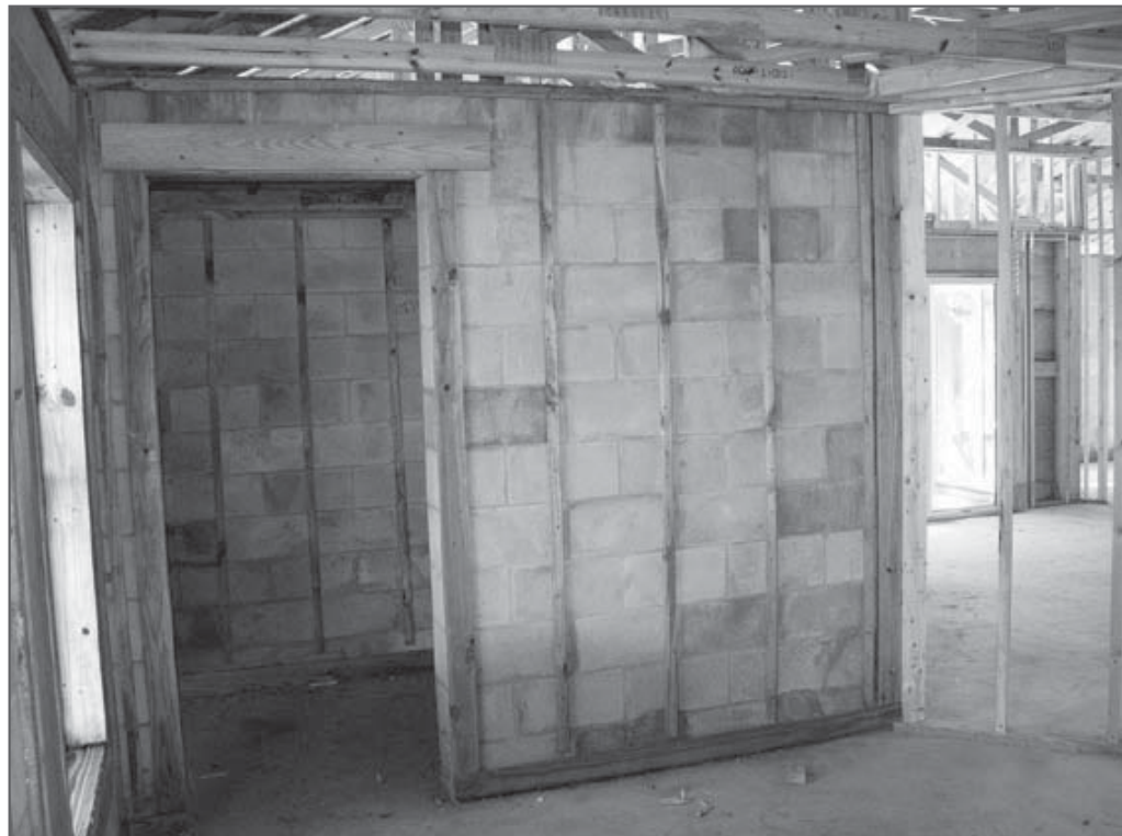
Figure II-6. View of an in-home safe room under construction. The CMU walls of this safe room are fully grouted and are reinforced, vertically, with steel reinforcing bars from the foundation to the concrete roof deck (New Smyrna Beach, Florida).
