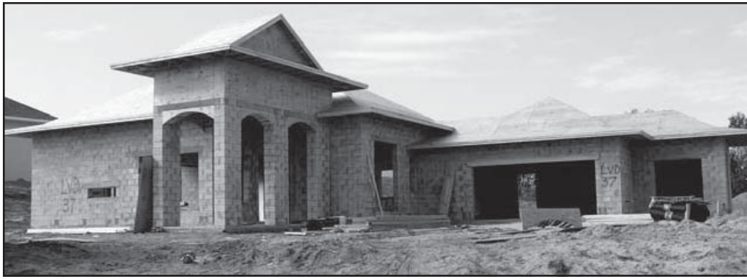
Figure II-5. CMUs were used for the exterior walls at this home under construction (New Smyrna Beach, Florida).
