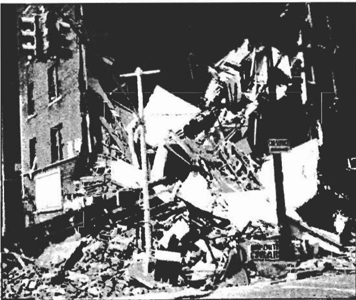
In photo above, the top floors reveal an unsupported lean-to collapse and the bottom exhibits a pancake collapse at August 1997 incident at 3851 Flatlands Avenue, Brooklyn.
