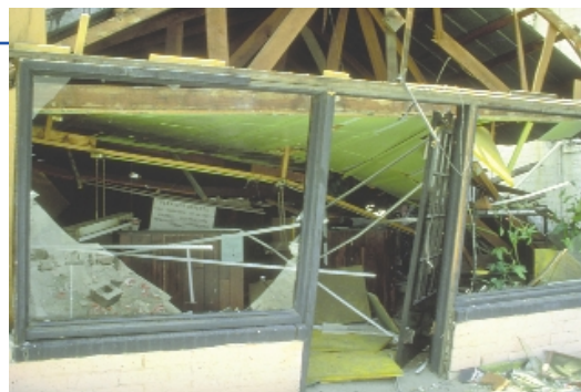
Damaged building, Coalinga, Calif.
