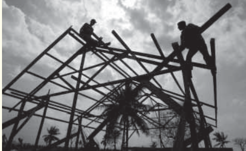
Workers Rebuild a House which was Destroyed by the Tsunami in Banda Aceh, Indonesia, on the One-Month Anniversary of the Disaster Wednesday, Jan. 26, 2005.
